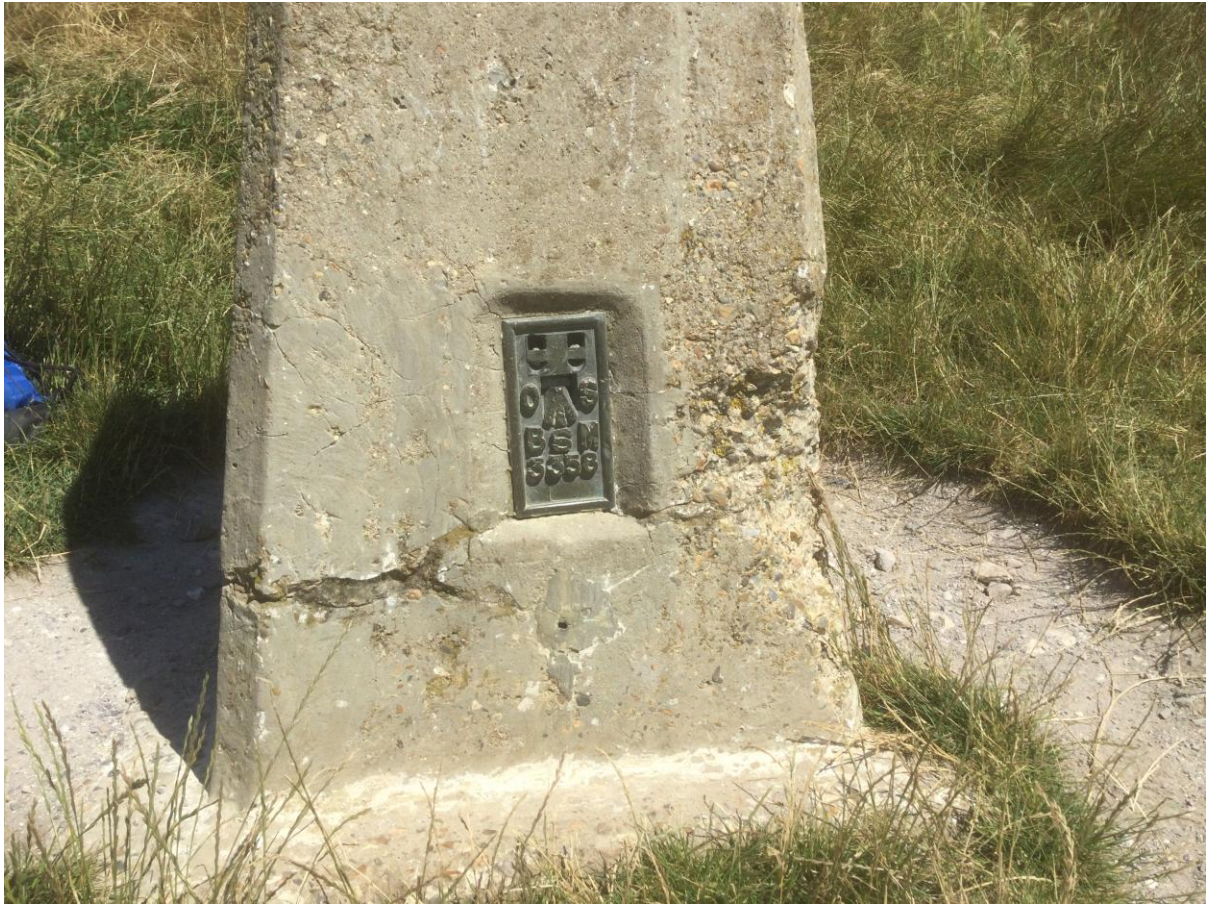
Damage to the Box Hill trig pillar
